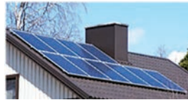
Figure 2.33 Solar cell panels
