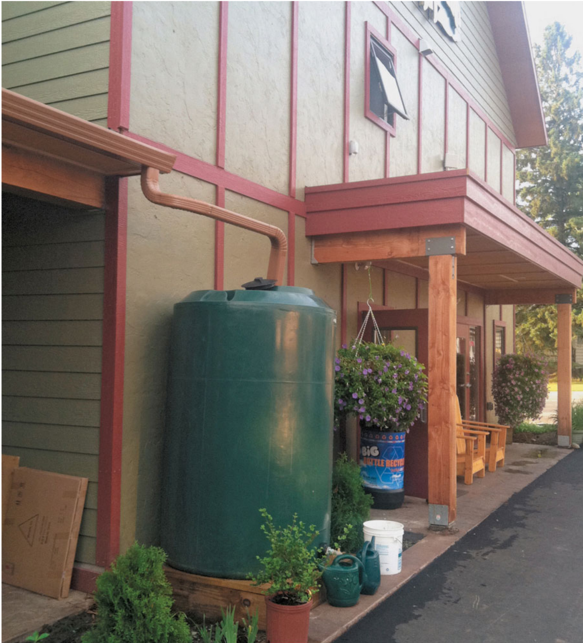
Larger rainwater harvesting systems can be designed to collect the maximum amount of water possible.
