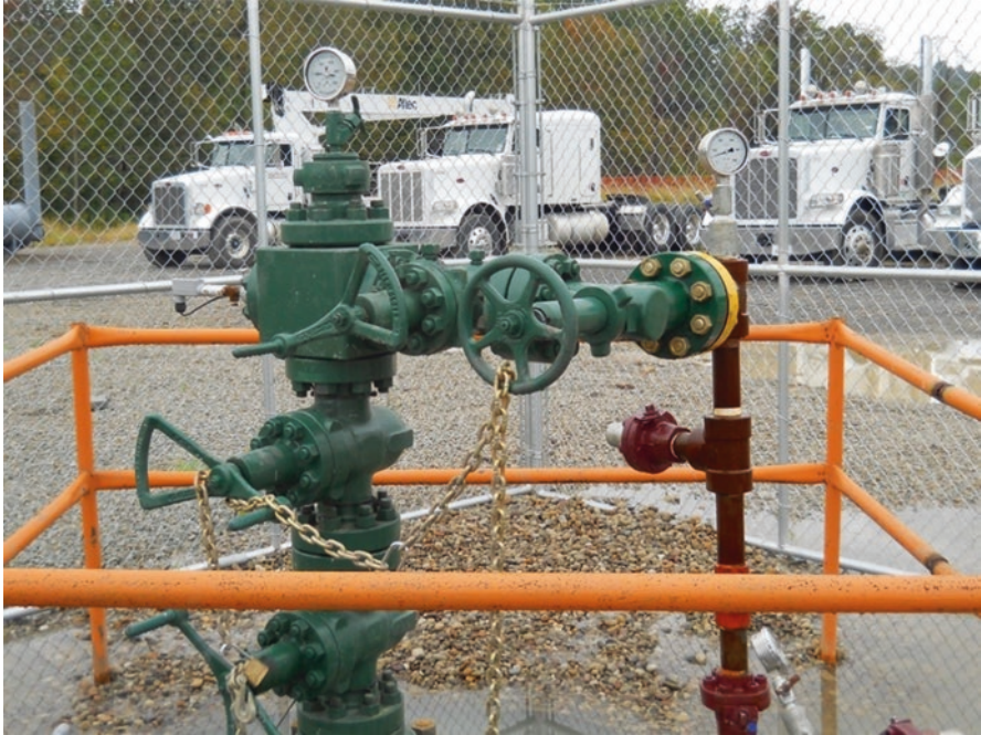
Fig. 2.6 A post-completion, production wellhead known as a “Christmas tree” installed on a shale gas well in Pennsylvania. (Photographed in 2012 by Dan Soeder)
