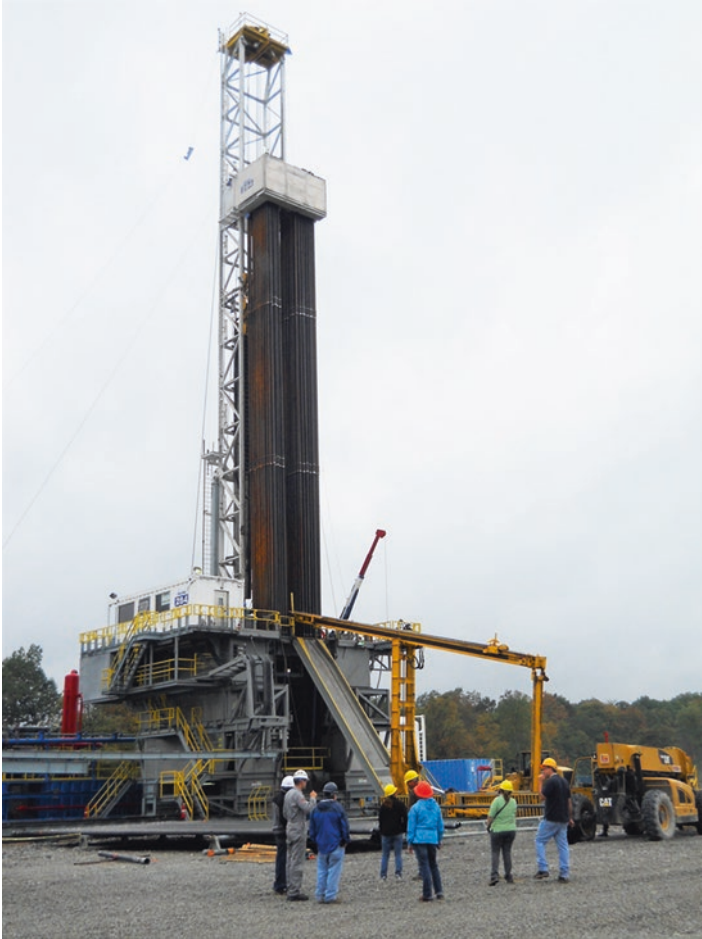
Fig. 7.1 A triple drill rig towers over both trees and visitors at a Marcellus Shale site in Pennsylvania. (Photographed in 2011 by Dan Soeder)
