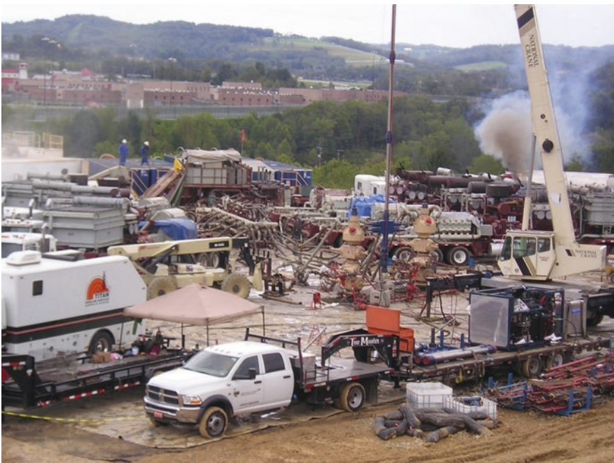
Fig. 2.5 Initiating a hydraulic fracture in the Marcellus Shale at a wellsite in southwestern Pennsylvania. (Photographed in 2011 by Dan Soeder)
