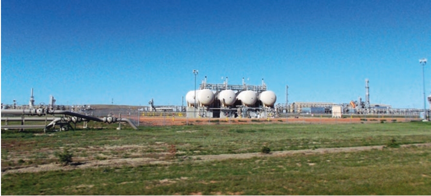
Fig. 7.4 A small segment of the sprawling ONEOK Garden Creek Plant for processing Bakken gas near Watford City, ND. (Photographed in 2017 by Dan Soeder)
