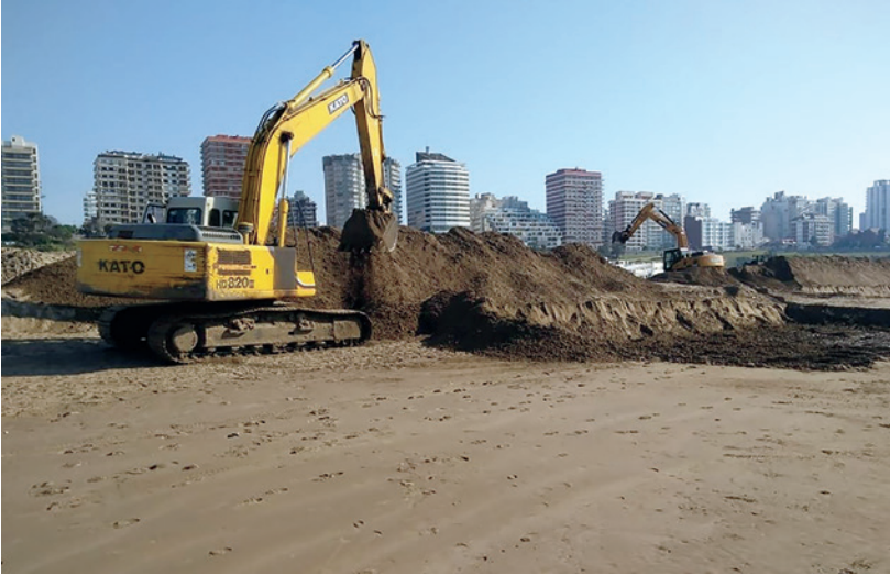
FIG 7.1 Sand mining along the Buenos Aires, Argentina, coast. Beaches provide raw material for construction, and the city skyline reflects the demand for aggregate sand. But this shouldn't be at the expense of loss of the beach. Photo courtesy of Federico Isla.
