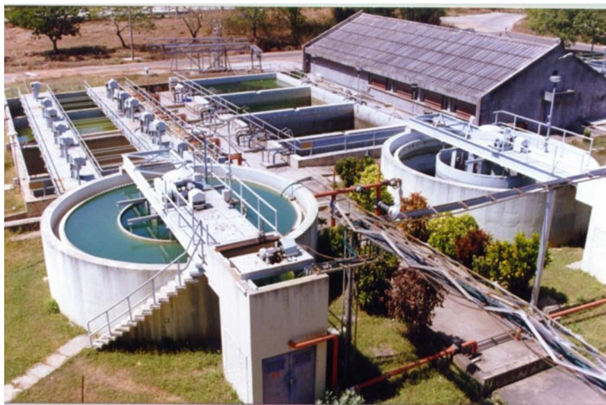
Fig. 8.2 Chemical treatment of LILW: settlers used for precipitation of sludges
