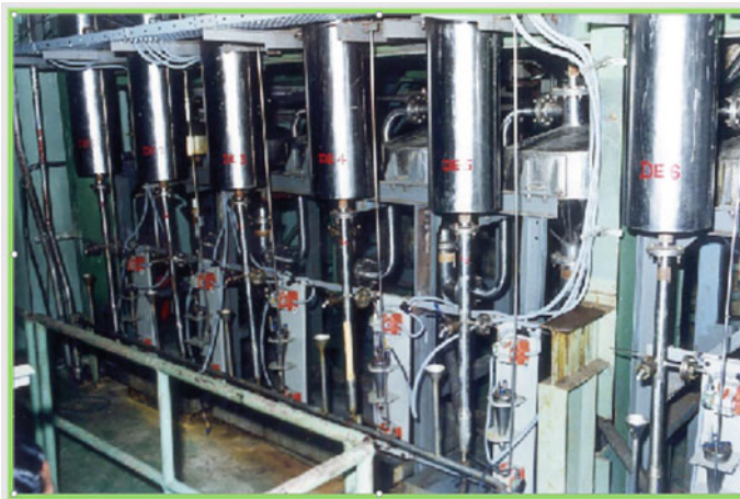
Fig. 2.14 Slurry extractor used in the Solvent extraction system
