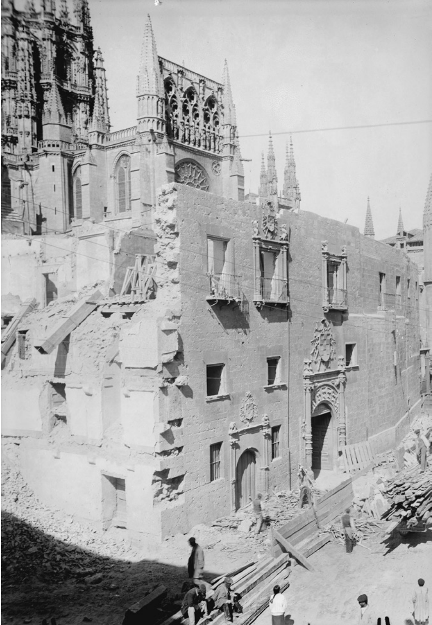
FIGURE 1 Old Episcopal Palace, Burgos, during demolition, ca. 1914 PHOTO: ARCHIVO MUNICIPAL DE BURGOS
