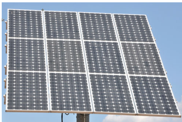
Fig. 55.3 Solar panels. (Photo Joaquim Sanz. MGVM)
