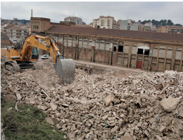
Fig. 85.5 Recovery of aggregates from the demolition of a building. (Image courtesy of Regió 7)
