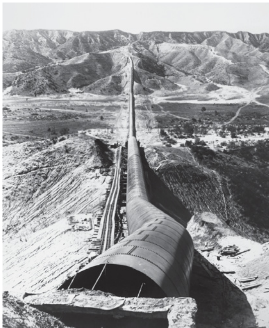
Fig. 5.2.6 Los Angeles receives much of its water from Owens Valley, 300 km to the north. The water negotiates the mountains and valleys in between, driven by gravity alone. Giant pipes allow pressure to build during downhill stretches to push the water back uphill later on. Parts of the 1913 aqueduct support so much pressure that the steel pipe used in them has to be more than an inch thick.
