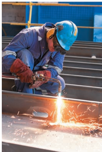
▲ Oxyacetylene Welding The reaction of oxygen and acetylene gases releases enough heat to melt iron.
