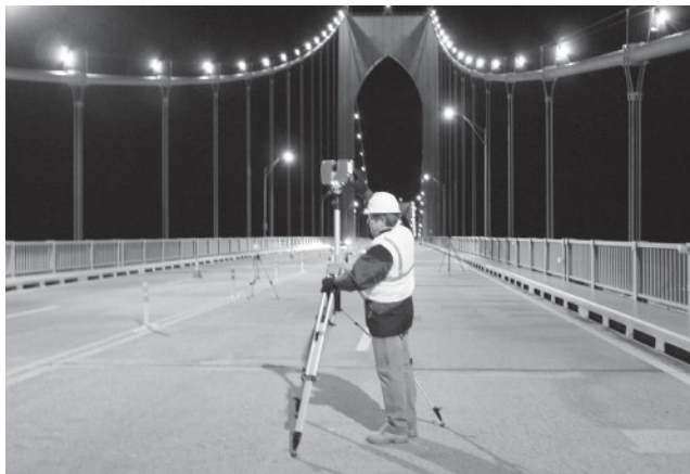
Figure 7.19 Adjusting scanner at fixed spacing intervals and heights to control scan density of road surface
