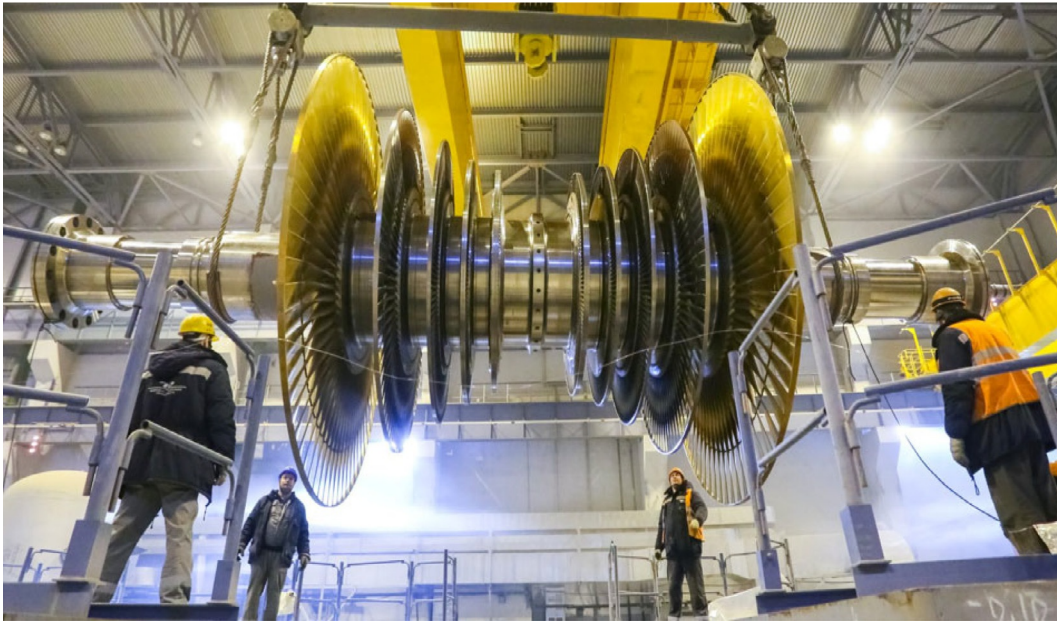
FIG. A1.62 Installation of double-flow low-pressure-turbine rotor with blades for VVER-1200 (Generation-III + ), 1066 MW el , Unit 2, Leningrad NPP, year 2018: https://www.flickr.com/photos/rosatom/40900768181/in/album-72157668094181020/ . Courtesy of Rosatom
