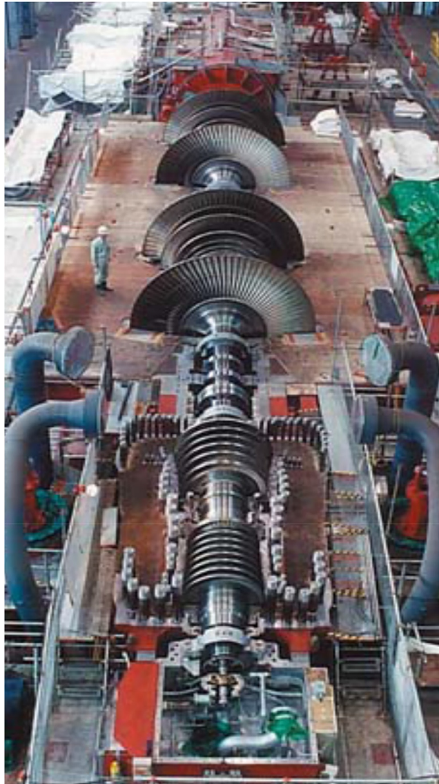
FIG. A1.14 Photo of Tomato-Atsuma (Japan) coal-fired-power-plant Unit No. 4 - supercritical-pressure steam turbine: 1 High-Pressure (HP), 1 Intermediate Pressure (IP) and 2 double-flow Low-Pressure (LP) cylinders: 700 MW e , TC4F-43, 3000 rpm, steam parameters - 25.0 MPa pressure and 600/600°C (primary steam/reheat) temperature. Courtesy and copyright by Hitachi, Ltd
