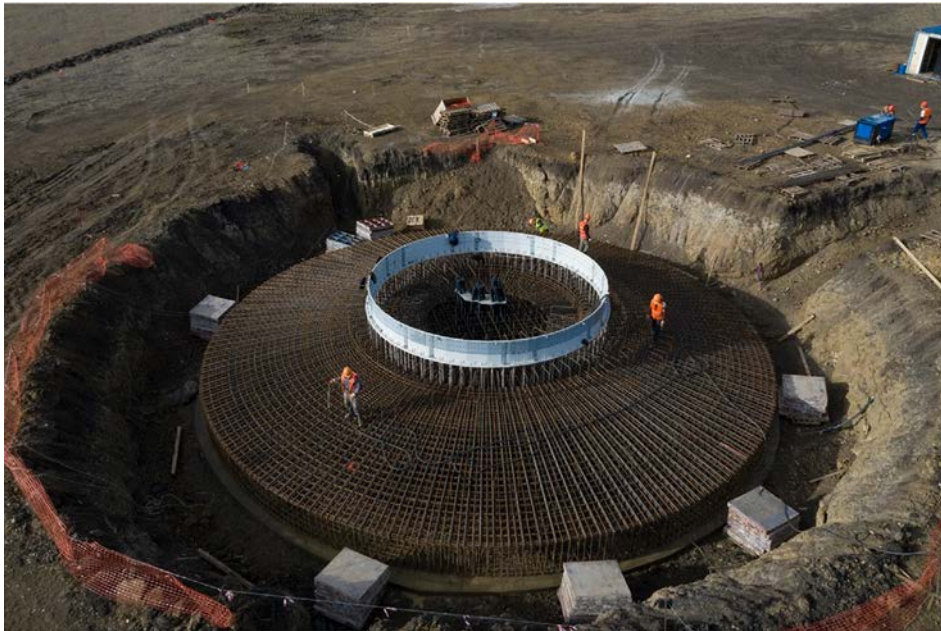
Figure 1.1.22b. Each wind turbine requires relatively large and heavy concrete foundation to withstand possible high winds and requires road access for servicing. Courtesy of Rosatom: https://www.flickr.com/photos/rosatom/50173267572/in/album-72157713699988403/
