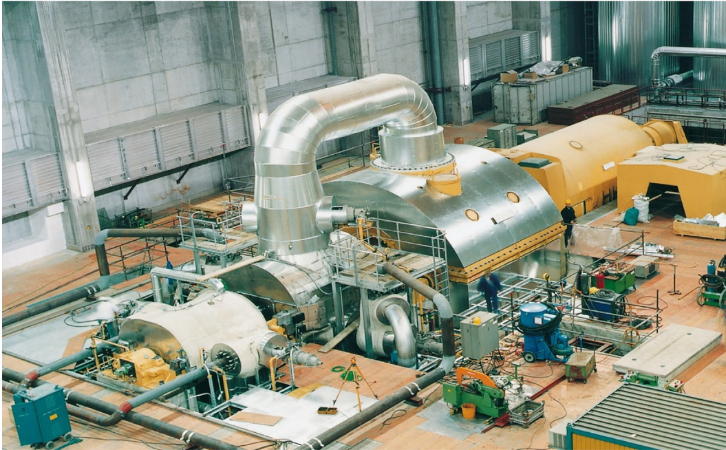
FIG. A1.9 Photo of 476-MW SST5-6000 steam turbine (barrel-type 1 HP, 1 double-flow IP and 1 double-flow LP cylinders) with hydrogen-cooled electrical generator (tandem arrangement) at cogeneration plant in Altbach, Germany. The plant can supply up to 280 MW th of district heat. Siemens press photo; copyright Siemens AG, Munich/Berlin, Germany
