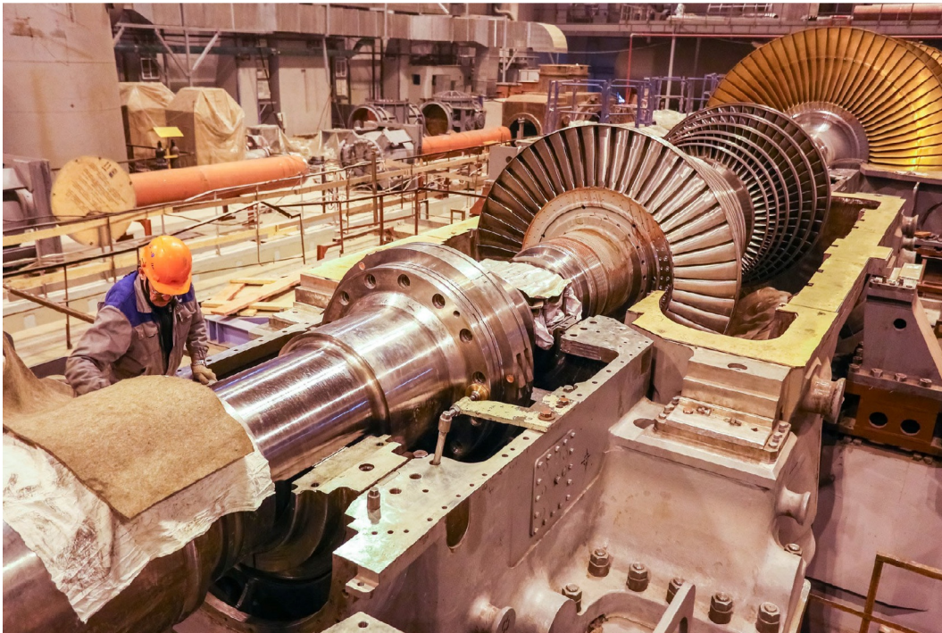
FIG. A1.61 Turbine assembling: From left to right – Shaft, double-flow high-pressure turbine and double-flow low-pressure turbine, VVER-1200 (Generation-III + ), 1066 MW el , Unit 2, Leningrad NPP. Courtesy of Rosatom: https://www.flickr.com/photos/rosatom/32216583188/in/album-72157668094181020/ ; Photo by S. Kashin/Titan-2, 2018
