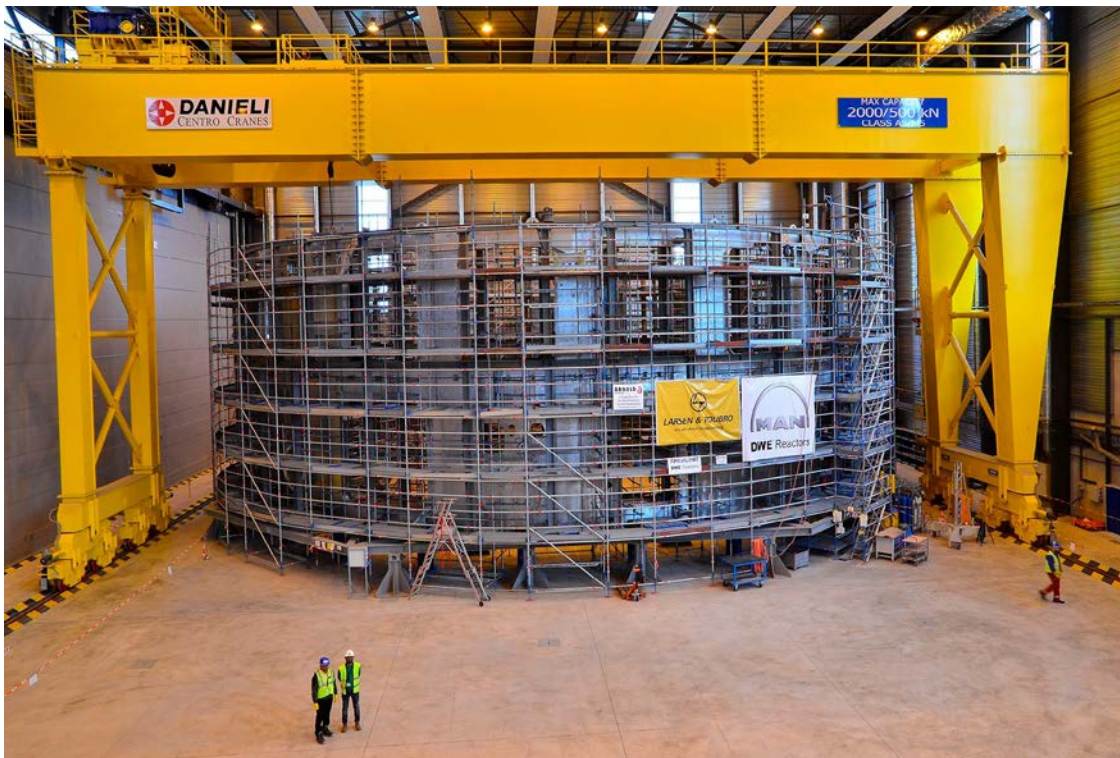
Figure 23.10. The base section of the ITER cryostat gives a good sense of the real size of the future reactor. The complete structure will be 30 m high. Weighing 1250 tons, it is the single heaviest component of the ITER machine. Credit: ITER Organization
