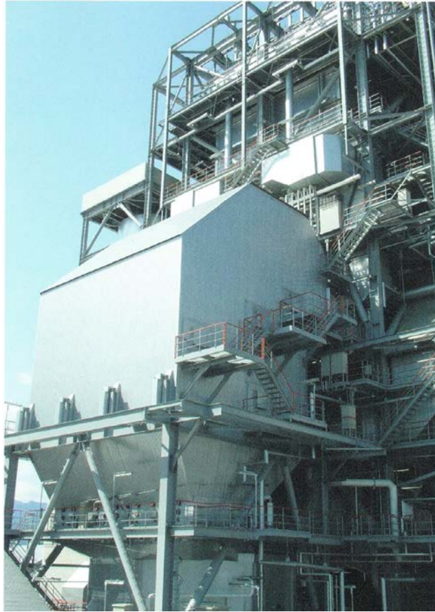
Figure 1.1.10b. Photo of thermal-power-plant Selective Catalytic Reduction (SCR) (DeNO x ) system with capacity of 746,000 nm 3 /h of exhaust gases. The SCR system helps to reduce NO x and CO emissions up to 96%. The DeNox system is based on the following reaction: 4\text{NO} + 4\text{NH}_3 + \text{O}_2 \rightarrow 4\text{N}_2 + 6\text{H}_2\text{O} . Courtesy and copyright of MHI
