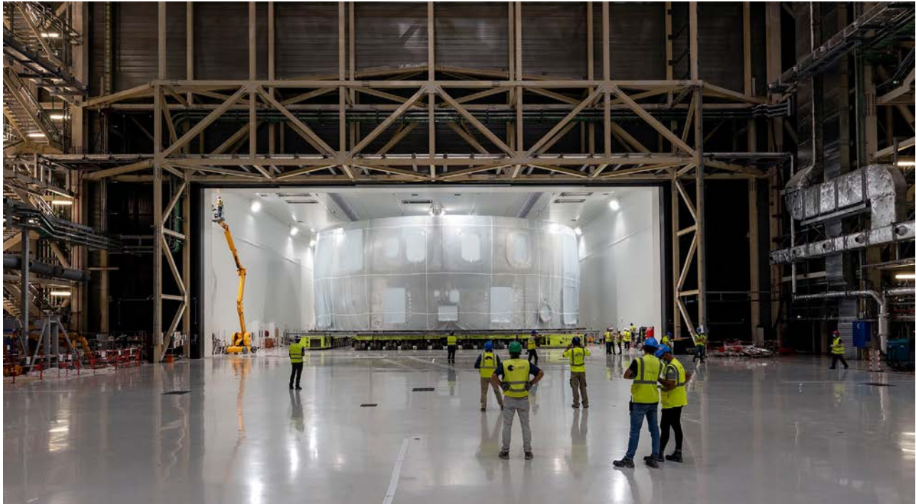
Figure 23.12. On August 22, 2020, the cryostat lower cylinder (lightly wrapped to protect it from weather, moisture and dust), 30 m in diameter and 375 tons, enters the Assembly Hall as it is transported out of the workshop by self-propelled modular transporter. Credit: ITER Organization
