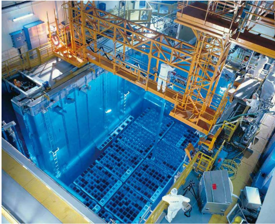
FIG. A1.31 Spent-fuel pool. HPC is currently moving through planning process to change interim-waste-storage method from wet store to dry store. Courtesy and copyright by AREVA (EDF)
