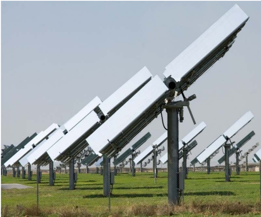
Figure 1.1.34. Photo of 1.2-MW el concentrated PhotoVoltaic (PV) solar-power plant (Spain). The plant has 154 two-axis tracking units, consisting of 36 PV modules each, which cover area of 295,000 m 2 with a total PV-surface area of 5913 m 2 . Plant generates 2.1 GWh annually. Conversion efficiency is 12%. Wikimedia Commons, author/username: afloresm
