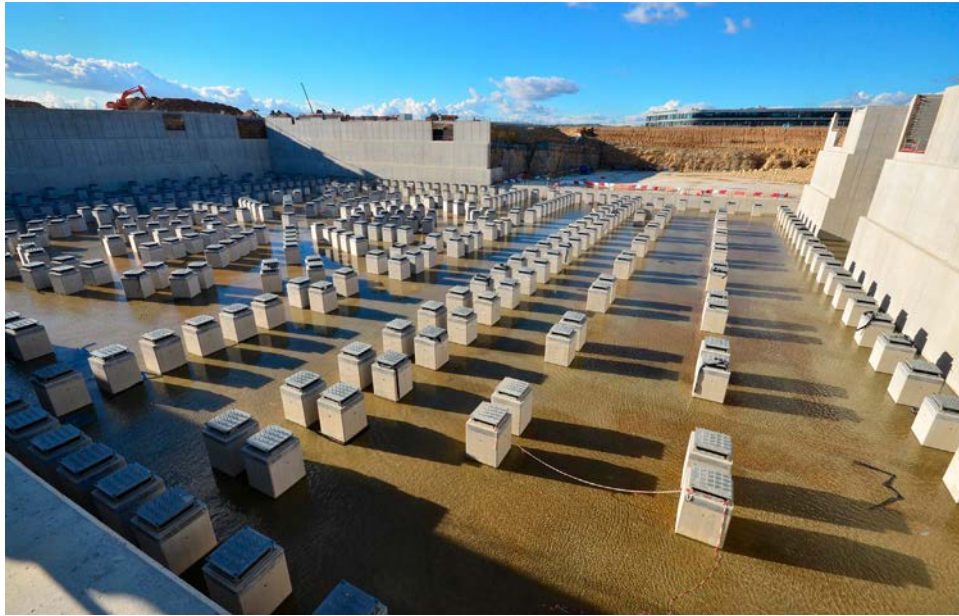
Figure 23.15. ITER’s ground support structure (photo taken on November 6, 2012). The 17-m deep, 1.5-m thick basemat, the retaining walls and the 493 separate columns constitute ITER’s seismic isolation pit. Credit: ITER Organization
