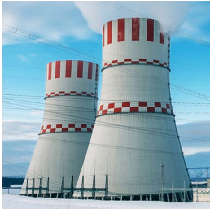
Figure 1.1.10c. Cooling towers. Courtesy of Rosatom: https://www.flickr.com/photos/rosatom/47368931231/in/album-72157672133127091/
