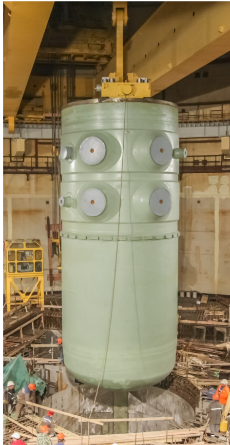
FIG. A1.49 Loading Reactor Pressure Vessel (RPV), 1100-MW e1 Unit 1 (Generation-III+), Leningrad NPP-2, year 2014: https://www.flickr.com/photos/rosatom/27143904732/in/album-72157668094181020/ . Large openings (850 mm ID) are for reactor-coolant flow in - lower level and out – upper level; smaller ID (300 mm) opening to the left upper level is for emergency cooling; and two pivots for crane for lifting RPV parts are shown: one to the left lower level and one to the right upper level with other two pivots 180° apart. Courtesy of Rosatom
