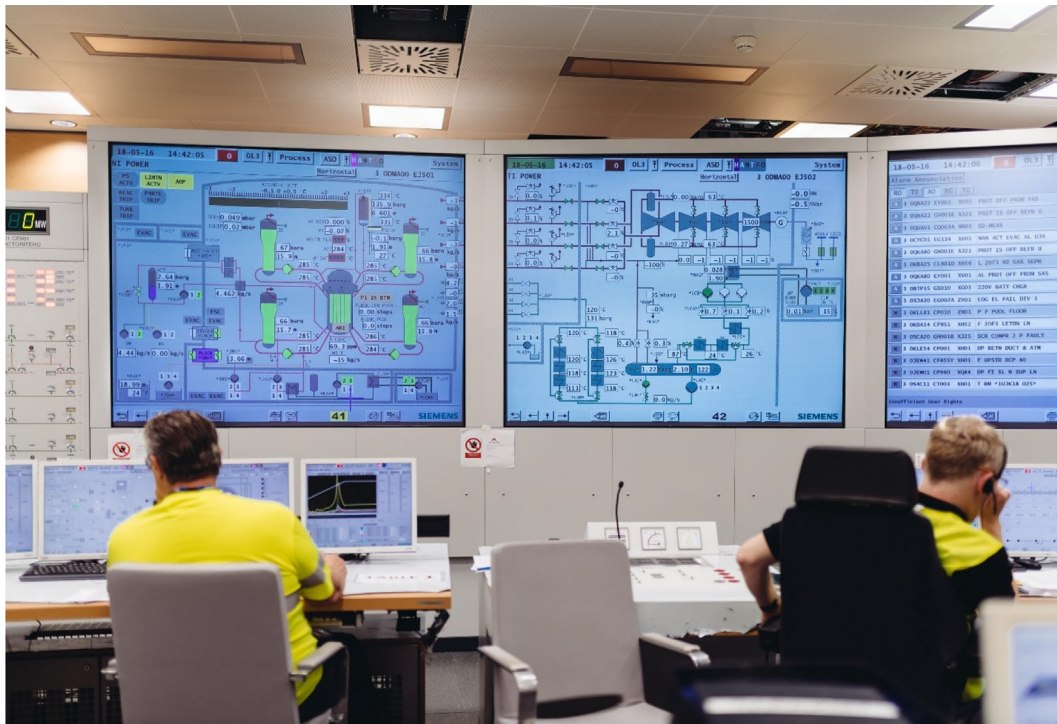
FIG. A1.35 Shown part of control hall: 1,600-MW el EPR, Olkiluoto NPP, Finland (connected to grid in March 2022). Courtesy of TVO (Teollisuuden Voima Oyj), Finland
