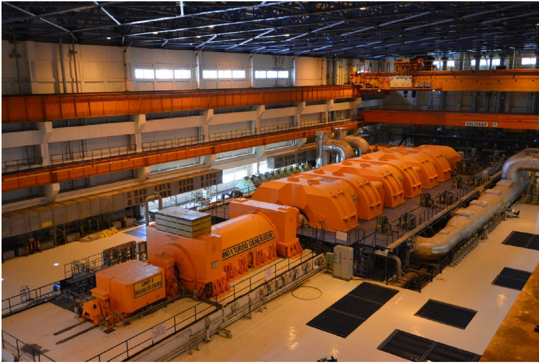
FIG. A1.60 Turbine-generator hall of Kudankulam NPP, Unit 2, VVER AES-92 (Generation-III), 932 MW el , year 2016. Courtesy of Rosatom: https://www.flickr.com/photos/rosatom/27048124128/in/album-72157674579625065/ ; Photo Press Service IK "ASE"
