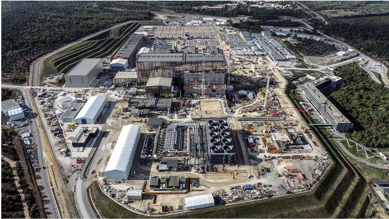
Figure 23.1. Aerial view of the ITER worksite in Cadarache (close to Marseille) in February 2022. The site has a total area of 181 ha (1,810,000 m 2 ). On the right side, the headquarters of the international organization (the bent building with a dark façade). The reactor will be located in the building surrounded by four cranes, which is next to the other tallest building on the platform (known as the “assembly hall”). Nearly 3000 people are currently working on the site. Credit: ITER Organization
