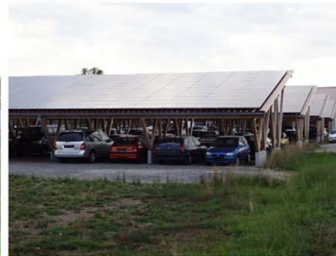
(c) photovoltaic panels installed on roof of parking lot.
