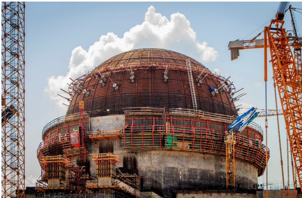
FIG. A1.59 Upper part of reactor containment building under final stages of construction, 1066-MW el VVER-1200 (Generation-III+), Unit 2, Leningrad NPP-2, year 2018. Containment building should withstand direct hit by airplane (intentional – terrorist attack or not intentional – air-accident): https://www.flickr.com/photos/rosatom/44271493640/in/album-72157668094181020/ . Courtesy of Rosatom
