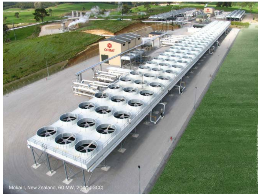
Figure 1.1.43b. Photo of Ormat air-cooled integrated geothermal combined-cycle power plant ( 60\text{MW}_{\text{el}} )—Mokai I, New Zealand. Courtesy of ORMAT, USA: http://www.ormat.com/geothermal-power
