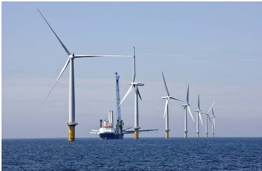
Figure 1.1.26b. Photo of off-shore wind park (power plant), Horns Rev. II (Denmark). The facility, located in the North Sea, has the maximum output of about 210 MW el ( 91 \times 2.3 MW el Siemens wind turbines), enough to meet the electricity needs of approximately 200,000 households. In general, as of today, offshore wind power plants are, at least, 2.5–3 times smaller by installed capacity than onshore wind power plants, but offshore wind turbines can be significantly larger by power and by a rotor diameter compared to that of onshore turbines (see Figure 1.1.26c ). Siemens press photo; copyright Siemens AG, Munich/Berlin, Germany
