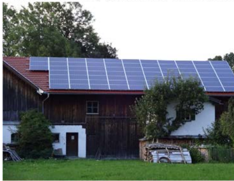
(b) photovoltaic panels installed on roof of house.
