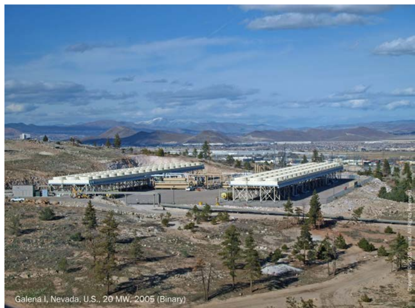
Figure 1.1.41b. Photo of Ormat air-cooled binary geothermal power plant (20 MW el )—Galena I, Nevada, US. Courtesy of ORMAT, USA: http://www.ormat.com/geothermal-power
