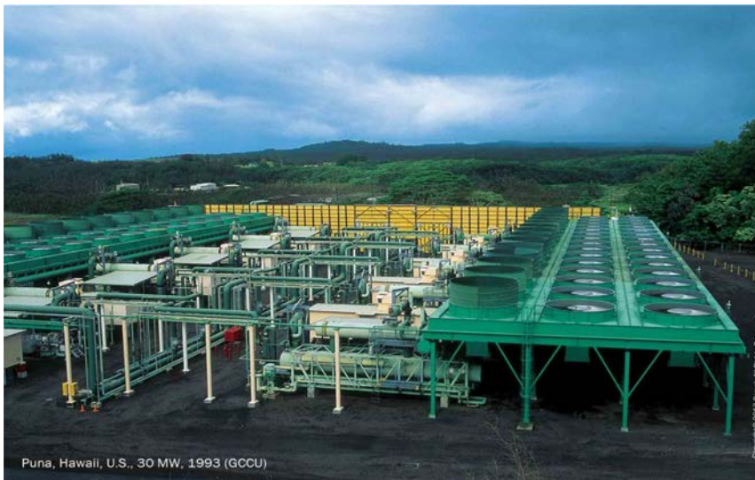
Figure 1.1.42b. Photo of Ormat air-cooled geothermal combined-cycle power plant (30 MW el )—Puna, Hawaii, US. Courtesy of ORMAT, USA: http://www.ormat.com/geothermal-power
