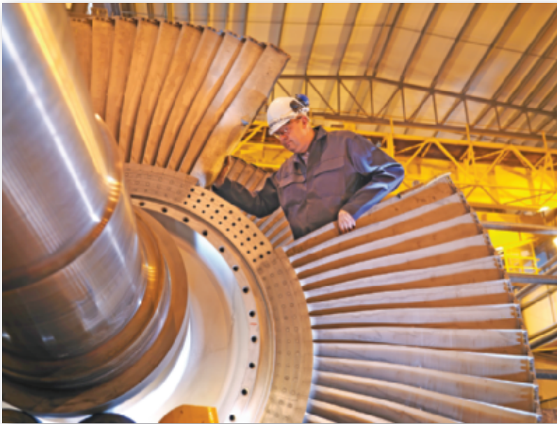
Maintenance of capital-intensive facilities requires good planning to minimize downtime. Here, turbine overhaul is under way. Organizing the thousands of parts and pieces necessary for a shutdown is a major effort.
