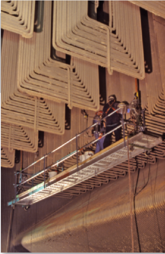
Two employees are on scaffolding near the top of Stanton Energy Center's 23-story high boiler, checking and repairing super heaters.
