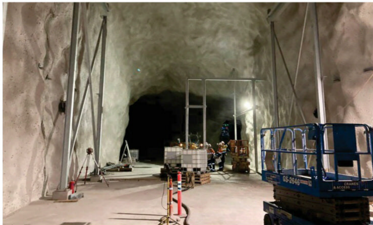
Rocky renovations: Turning a mine into a lab's a multi-year process, coating rocks and finding ways to minimise dust and humidity.
