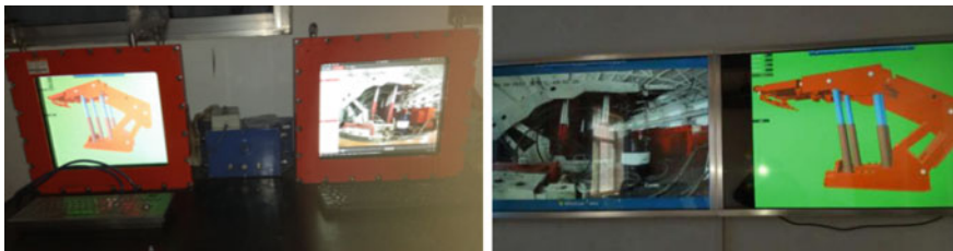
Fig. 11.9 Centralized control center test and remote dispatch center test
