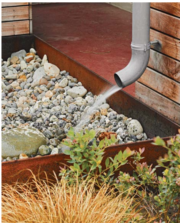
above • A downspout pours into the beach stone dry well, right into the soil below. This way, it can water the nearby plants and replenish the aquifer, deep below the surface.
