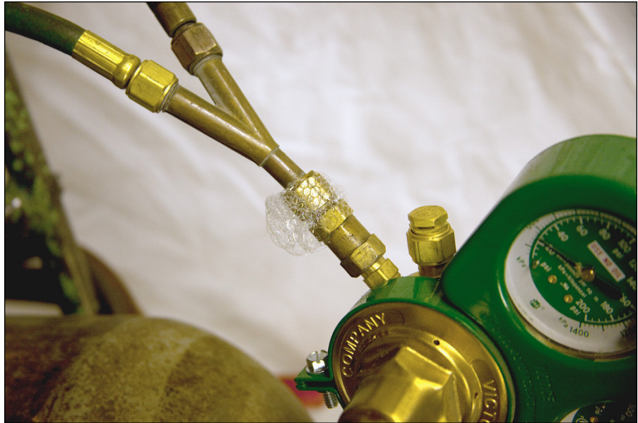
FIGURE 3-4: An example of a leaking oxygen hose.
