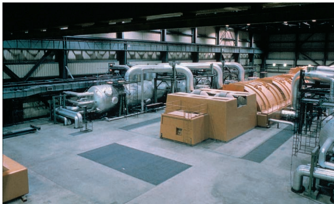
FIGURE 13.18 The turbine deck of a nuclear generating station. There is one large generator in line with four steam turbines in this nonnuclear part of the plant. The large silver tanks are separators that remove water from the steam after it has left the high-pressure turbine and before it is recycled back into the low-pressure turbines. Source: © Arizona Public Service Company.
