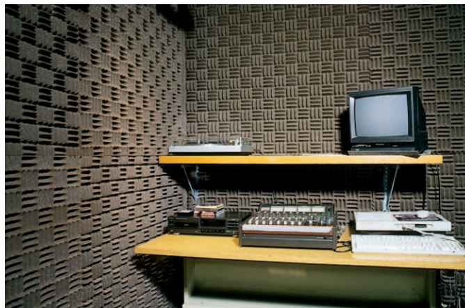
FIGURE 5.14 This closed-circuit TV control room is acoustically treated by covering the walls with sound-absorbing baffles. Reverberation and echoes cannot occur in this treated room because absorbed sounds are not reflected. Source: © McGraw-Hill Education/Bob Coyle.
