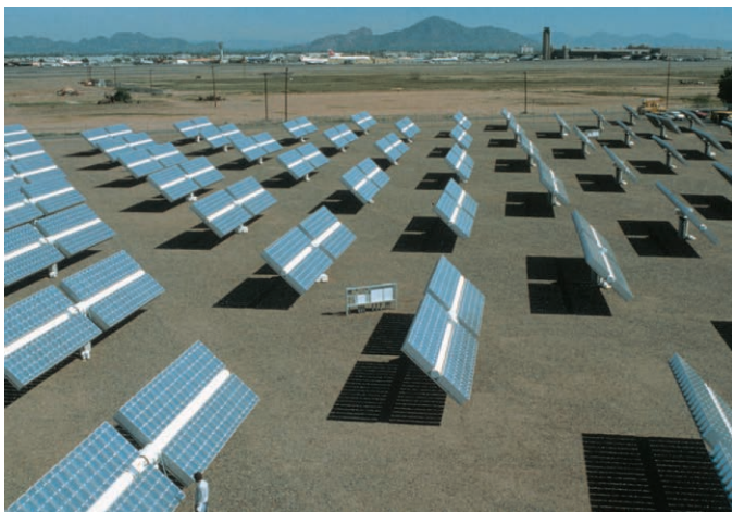
FIGURE 3.13 This demonstration solar cell array converts radiant energy from the Sun to electrical energy, producing an average of 200,000 watts of electric power (after conversion). Source: © Arizona Public Service Company.
