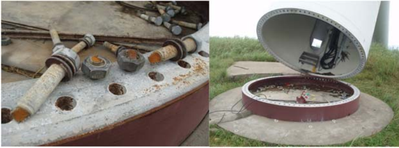
FIGURE 12.12 Damages to the connections due to hurricane Saomai.
