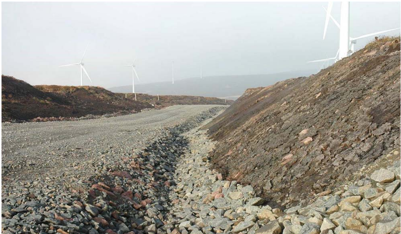
FIGURE 30.18 Newly constructed tracks cause ground disturbance. Photos: M van Grieken. All rights reserved.
