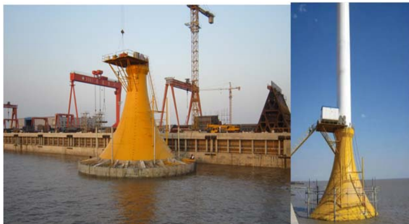
FIGURE 12.6 Large scale prestressed concrete bucket foundation in water depth of 6 m (the caisson dimensions are 30 m in diameter and 7 m in depth).
