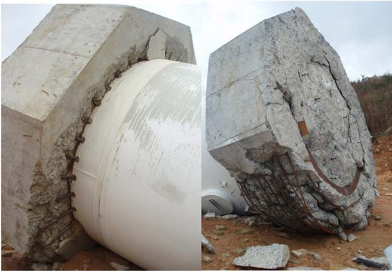
FIGURE 12.13 Damages to the foundations due to hurricane Saomai.
