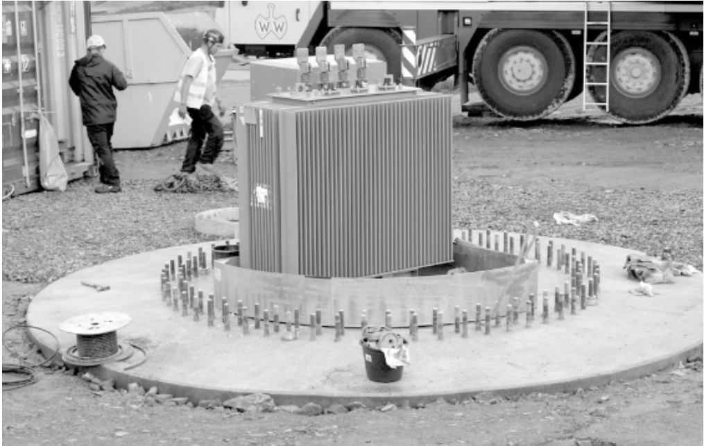
Figure 9.29 Transformer for an 800 kW wind turbine. The lowest tower section will be lowered into place over the top of the transformer, with the control cabinets installed in a floor immediately above.
