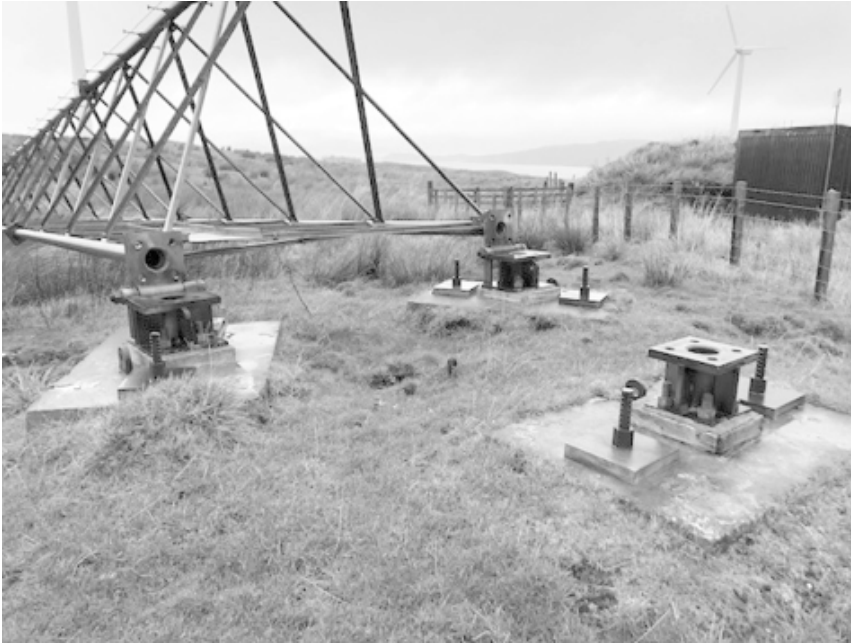
Figure 9.19 Hybrid rock anchor foundations. Each leg of the hinged lattice tower attaches to an individual reinforced concrete plinth, which is pinned to bedrock by two 6 m rock anchors. Demonstration project on the Island of Luing, Scotland. (Photo courtesy Shane Cadzow)
