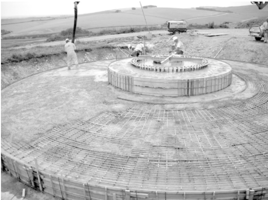
Figure 9.17 Construction of a slab-and-pedestal foundation for an Enercon E48. Concrete is being poured into the reinforcing cage; note the captive tower bolt ring rising out of the central pedestal. Once the foundation has been back-filled, only the pedestal will remain visible.
