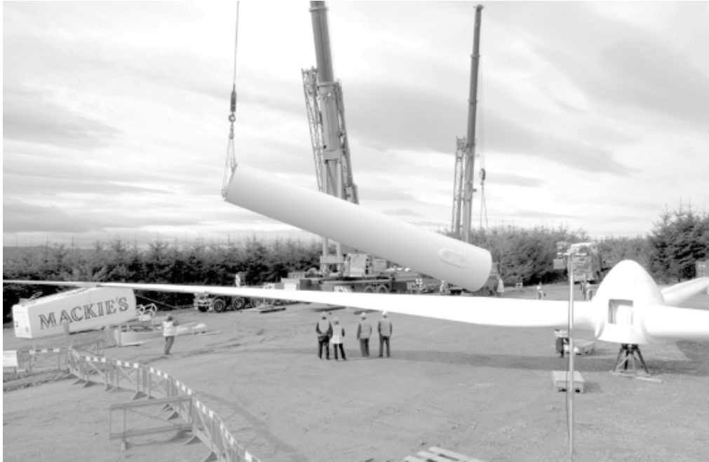
Figure 11.5 Construction of Mackies 850 kW on-site wind turbine. (Photo reproduced with kind permission of Mackies Ltd)
