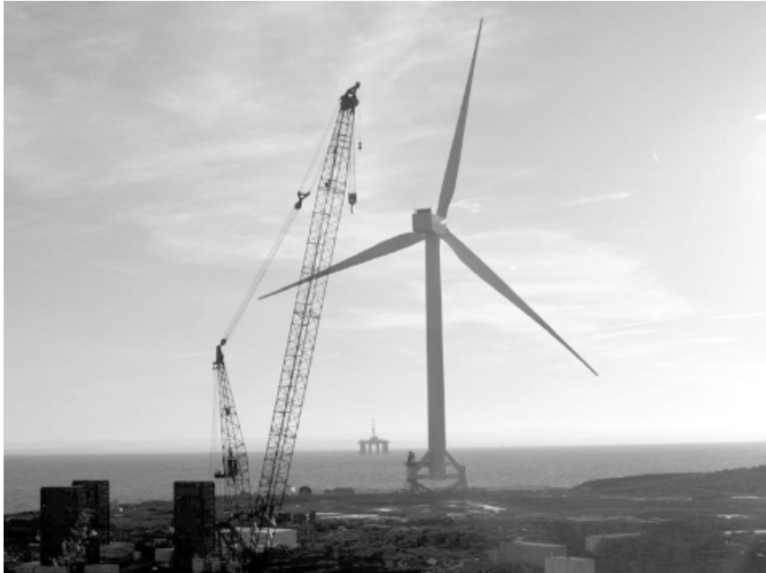
Figure 8.34 Samsung S7.0 wind turbine at Methil, Fife, on the east coast of Scotland. The rotor diameter of 171 m was the world's largest when installed in 2014 but has now (inevitably) been superseded.
