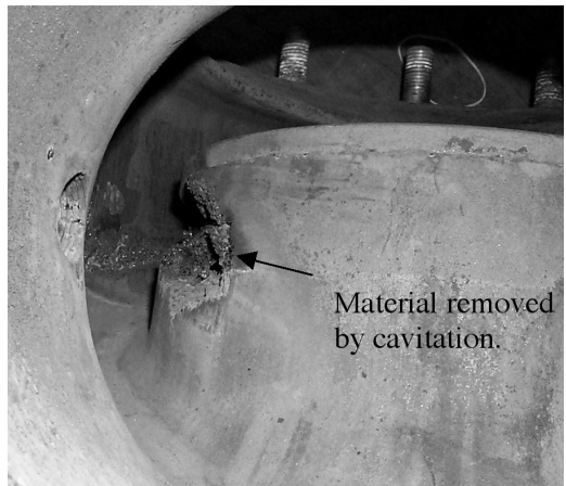
FIGURE 40.11 Cavitation damage in a globe valve (view from the downstream end of the valve).
